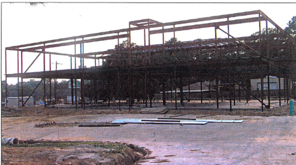
HOSPICE HOME: Construction continues on The Carpenter House, a $4.5 million facility at 10615 Jefferson Hwy., that will offer in-patient hospice service as well as serve as the new offices for St. Joseph Hospice. The two-story, 16,400-square-foot building is scheduled to open by the end of the year. Stuart Construction is the contractor.
